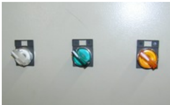
Picture 1.4. Replenishing / emptying control switches
