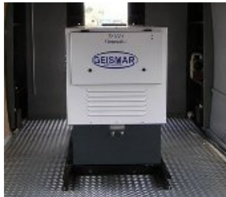
Picture 1.2. Diesel Generator.
