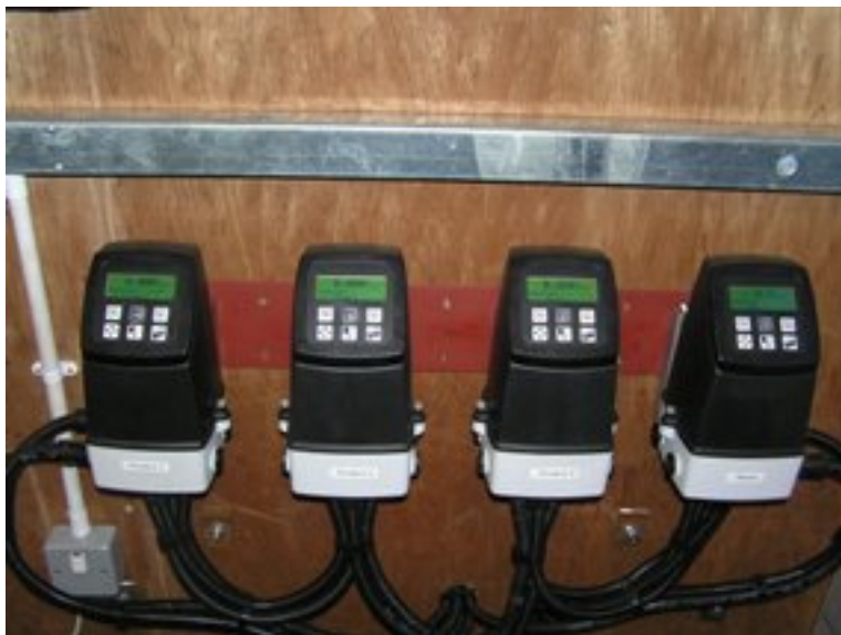
Picture 1.6. Flow meter displays.
