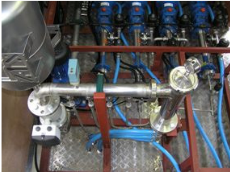
Picture 1.5. The chemical mixing system.
